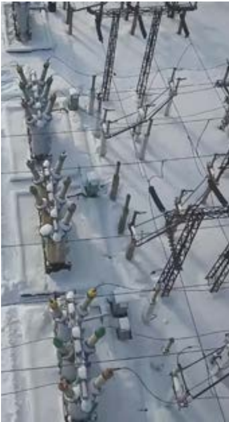
An electric substation in Kazakhstan. (Hlopotov/ Getty Images)
