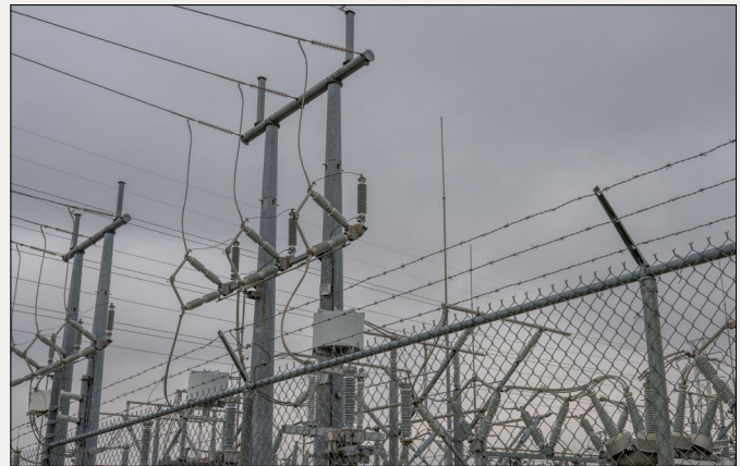
Transmission lines and towers sit behind barbed wire near the Energy Research Park in Houston, Texas. (Brandon Bell/Getty Images)
