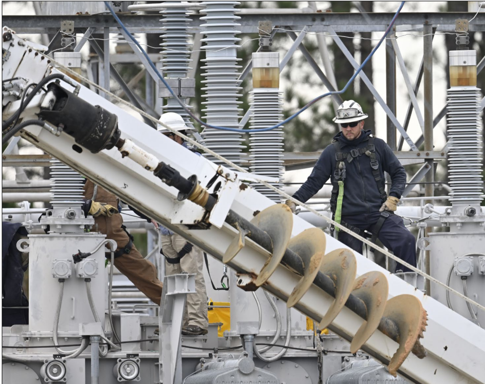
A worker repairs damage following an attack on power substations in Carthage, N.C., in December 2022. (Peter Zay / Anadolu Agency via Getty Images)
