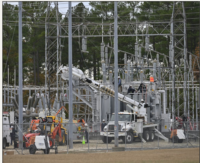
Workers repair damage following an attack on two Duke Electric power substations in Carthage, N.C. The attack left tens of thousands without power in Moore County on Dec. 05, 2022. (Peter Zay / Anadolu Agency via Getty Images)
